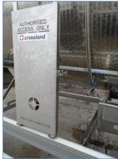
Ladder restriction with padlock and cable tie for cable system
