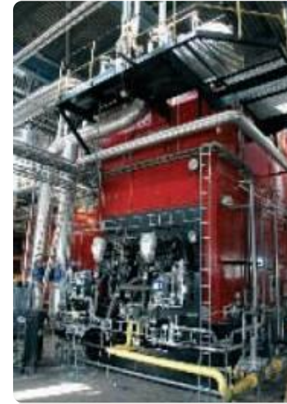
Bio-oil Boiler 1,200t
